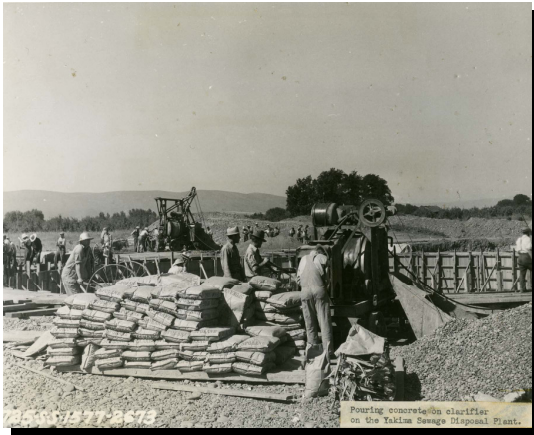
Yakima's original wastewater treatment plant cost about $315,000 and took about two years to build.
