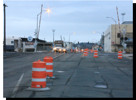
MLK, Jr. Blvd between 1 st Avenue and 1 st Street will be closed while a railroad underpass is built there.
